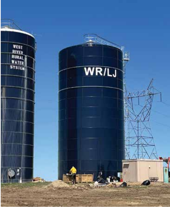
Completion of the new Creighton GSR (right).
